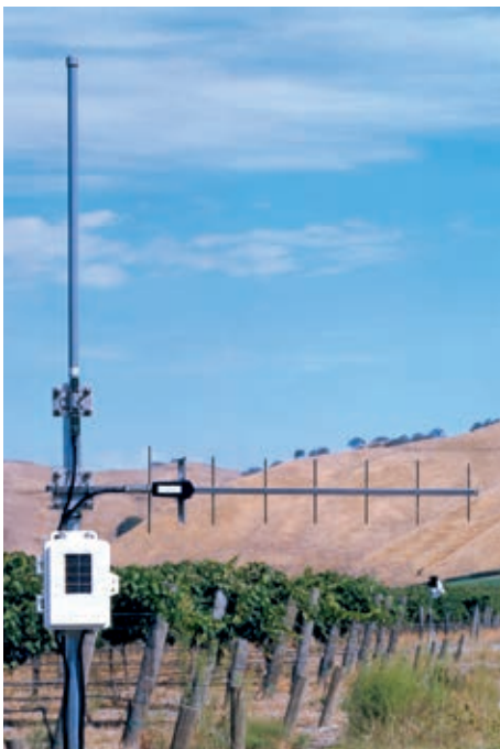
Long-range repeater with 1 Yagi and 1 Omni antenna.
